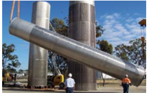
High-capacity vessel internals
